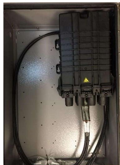
CommScope GCO2 with service loop
